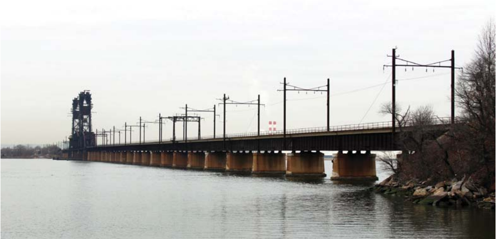
Northwestward view of the 4,005-foot, 31-span Newark Bay Bridge completed by the PRRC and LVRRCNJ in January 1930. CHRS, Inc. photograph, January 31, 2020.
